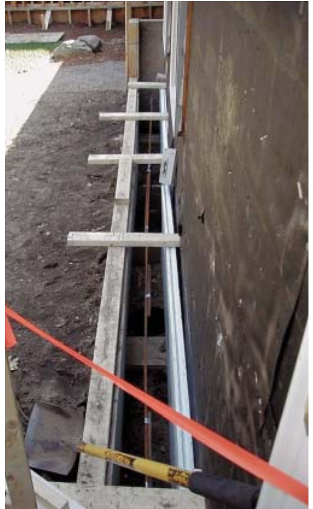
Figure 9. A new grade-beam concrete foundation, poured directly along the existing basement wall, and new wall framing provided direct support to eliminate the overhang of the second-story eaves wall.
