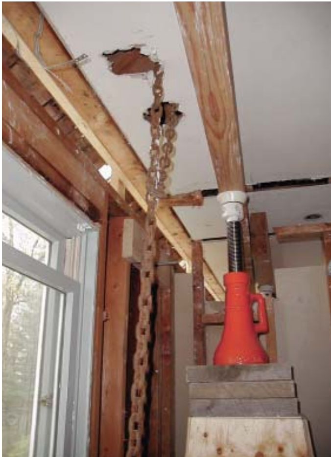
Figure 8. As a precaution against sudden strong gusts of wind, the crew tied the front and back of the house to the first story with a pair of heavy chains.
