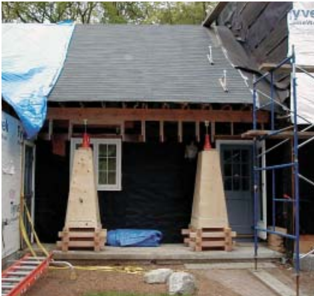
Figure 11. The screw jacks were limited to a 10-inch lifting range, so the jacking stands had to be supplemented with 4x4 cribbing placed in crosswise layers under the base.
