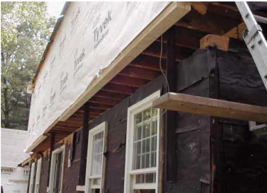
Figure 7. To prevent the upper story from being displaced when it was lifted, the author installed 4-inch steel angles to restrain it (above). At the overhanging front elevation (left), the crew cut L-shaped slots for the angles to pass through the second-story floor (below).
